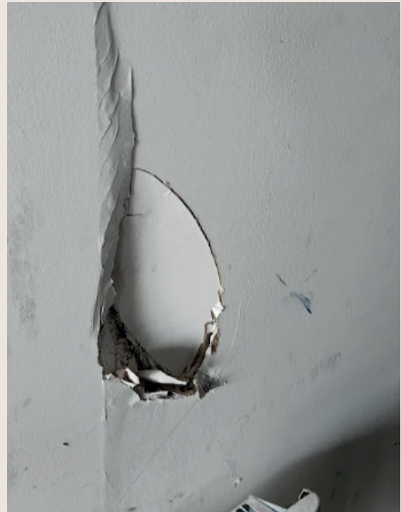
Figure 9. Damage to gypsum boards used for encapsulation
