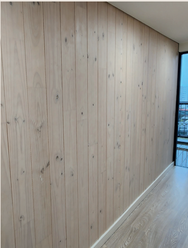
Figure 1. Exposed timber wall linings in non-sprinklered crowd use spaces may require a fire-retardant treatment (Credit: E. Claridge)
