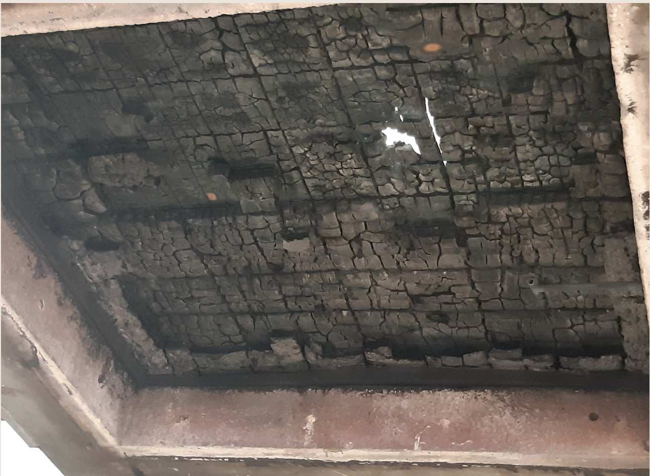
Figure 2. Example of char fall-off on the underside of a CLT slab during a fire resistance test (Credit: E. Claridge)
