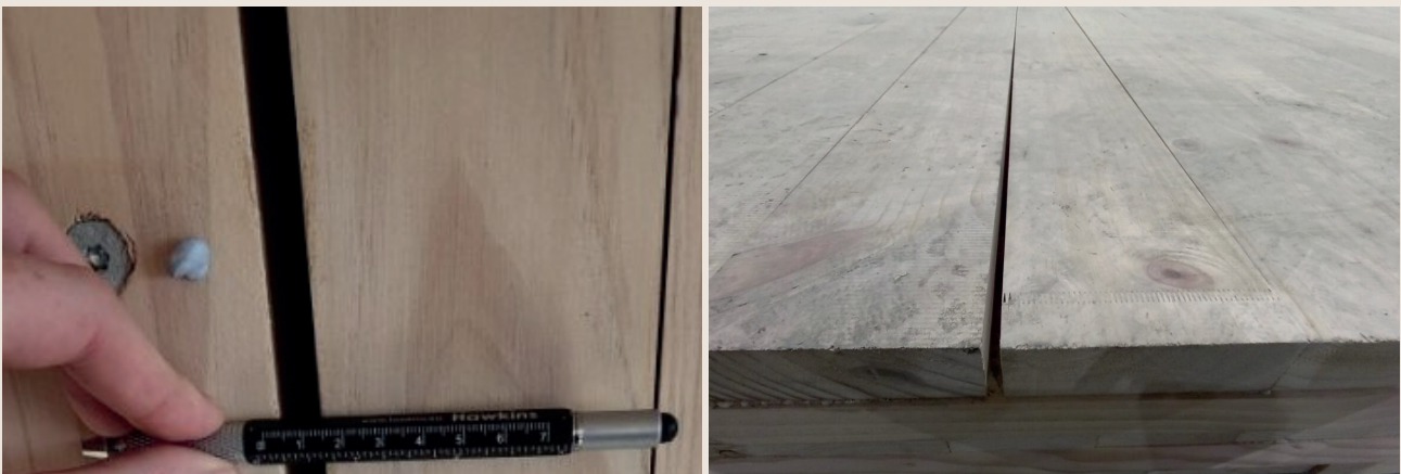
Figure 10. Gaps observed within premanufactured CLT panels after delivery to site (Credit: E. Claridge)
