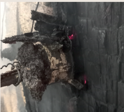
Figure 8. Ongoing burning behind a service penetration at the end of a fire test (Credit: E. Claridge)
