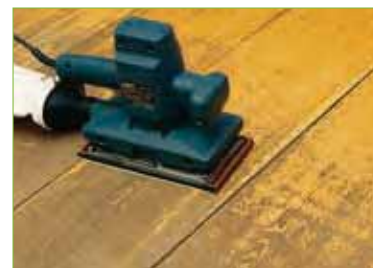
To renovate a floor, the lacquered surface must first be sanded down.
